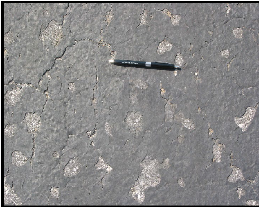
Figure A-199 High-Severity Raveling (Slurry Seal/Coal Tar Over Dense Mix)
