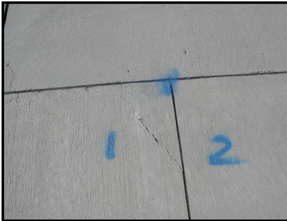
Figure A-278 Low-Severity Corner Spall
