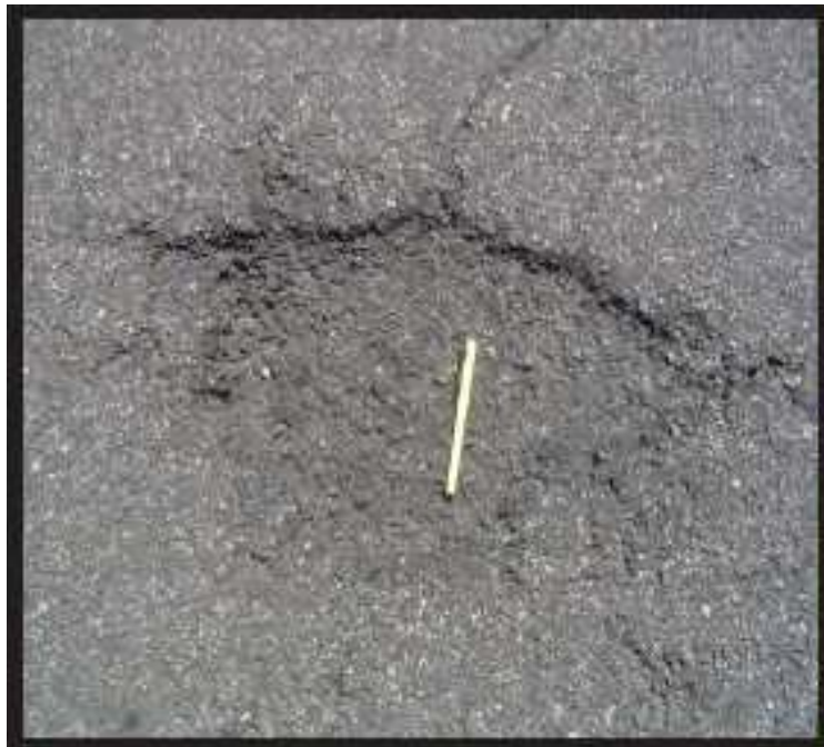
Figure A-48 Low-Severity Pothole
