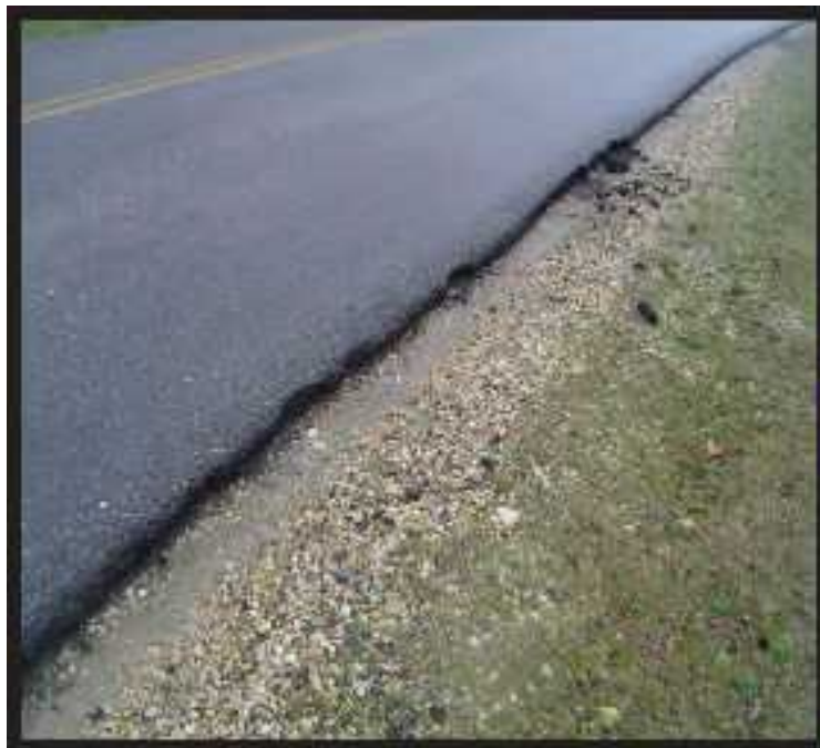
Figure A-34 Low-Severity Lane/Shoulder Drop Off
