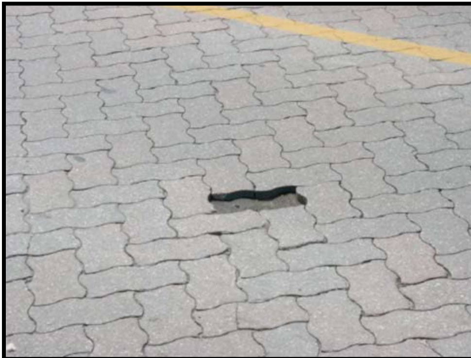
Figure A-332 Low-Severity Missing Pavers
