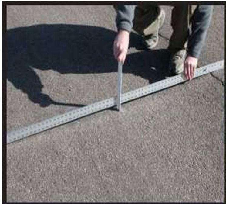
Figure A-22 Low-Severity Depression.
