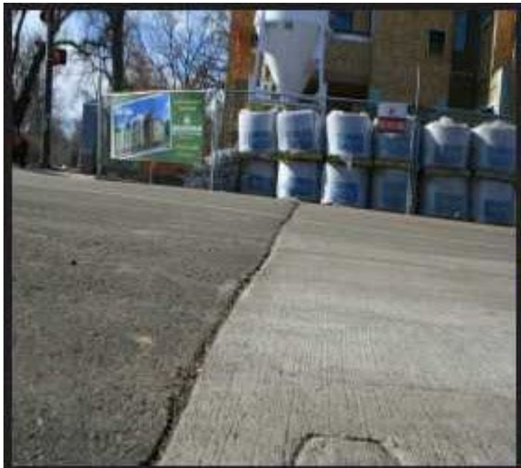
Figure A-60 Low-Severity Shoving
