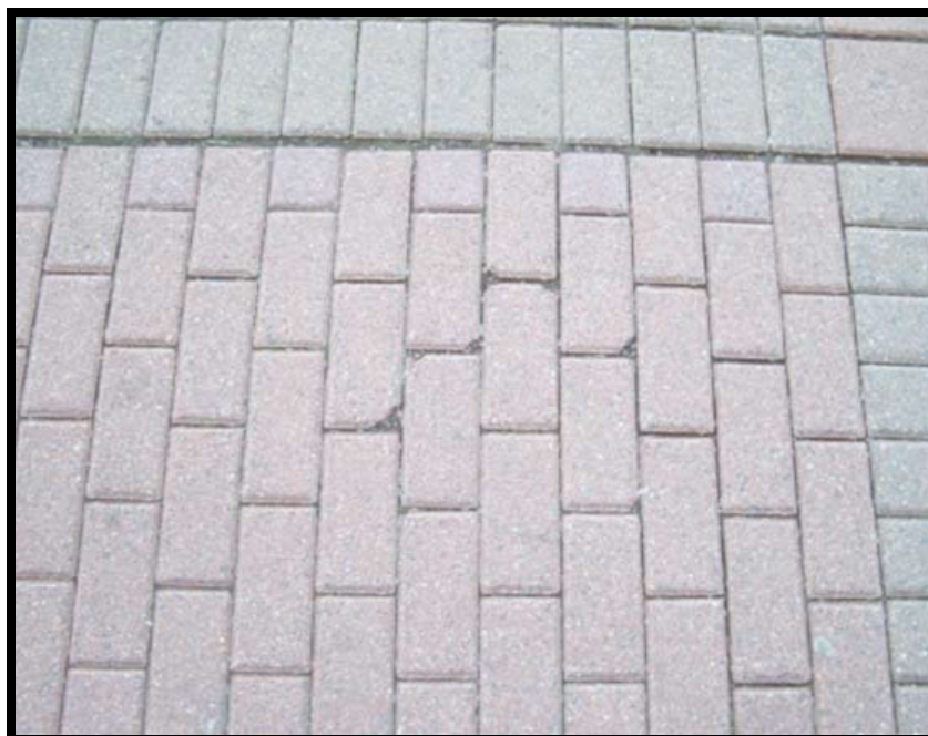
Figure A-300 Low-Severity Damaged Pavers
