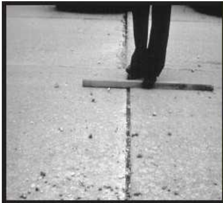
Figure A-94 Low-Severity Faulting
