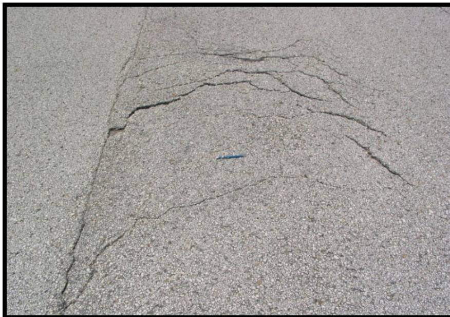
Figure A-213 Slippage Cracking
