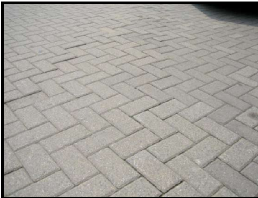
Figure A-316 Low-Severity Faulting
