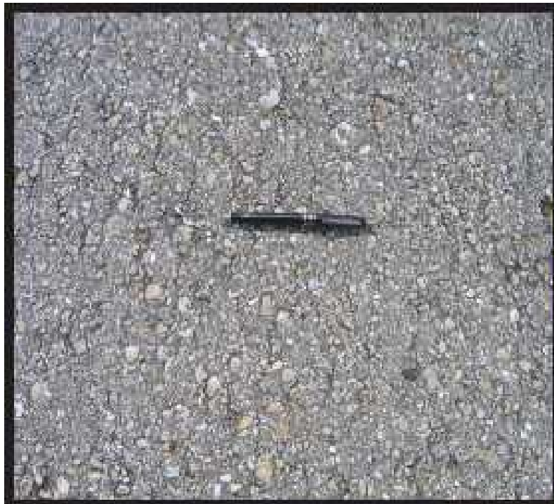
Figure A-73 Low-Severity Weathering
