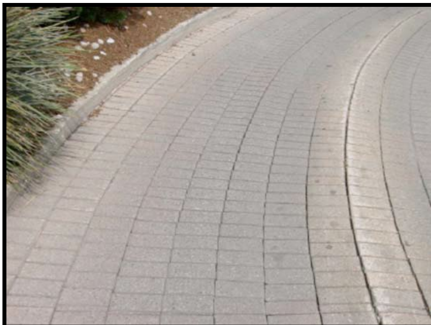
Figure A-340 Low-Severity Rutting
