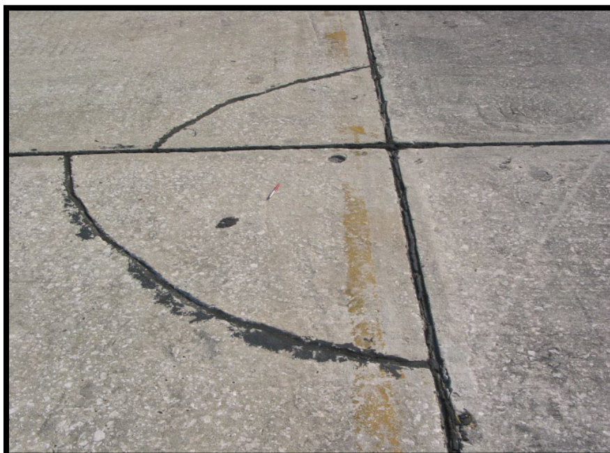
Figure A-229 Low-Severity Corner Break
