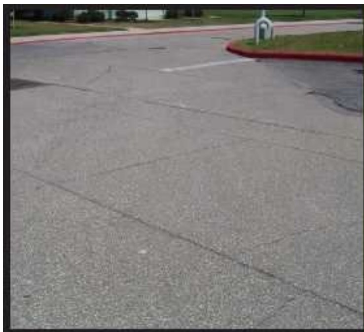
Figure A-30 Low-Severity Joint Reflection Cracking
