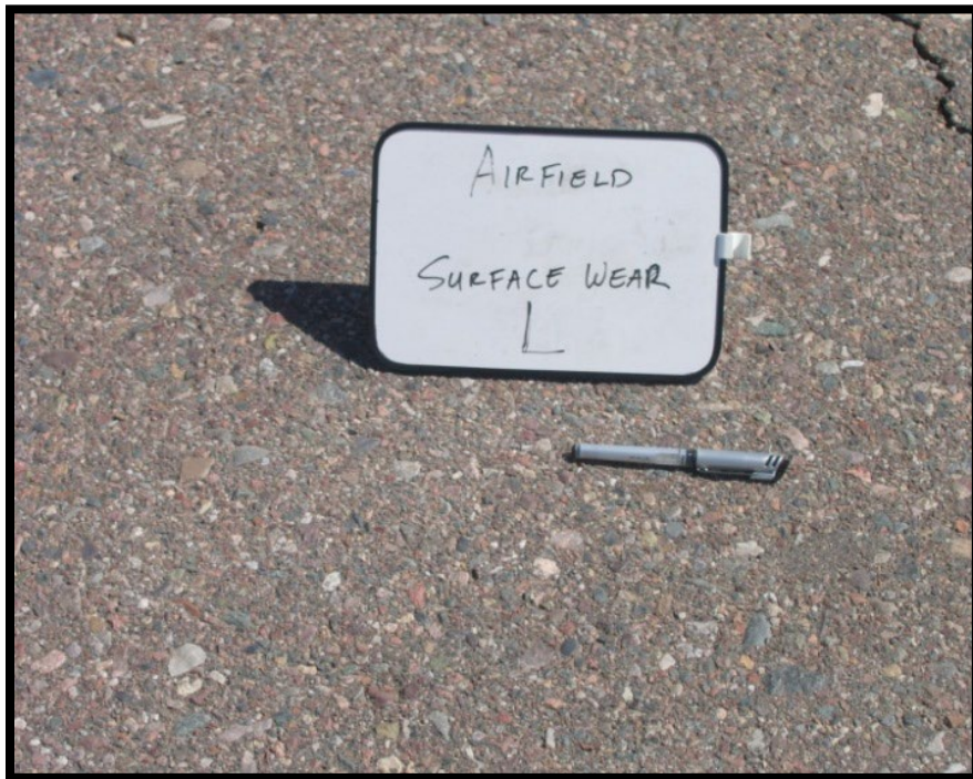
Figure A-219 Low-Severity Weathering
