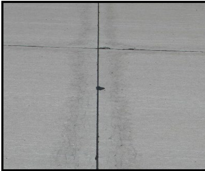
Figure A-238 Low-Severity “D” Cracking
