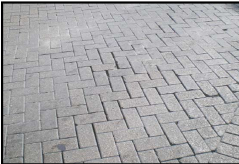
Figure A-324 Low-Severity Horizontal Creep
