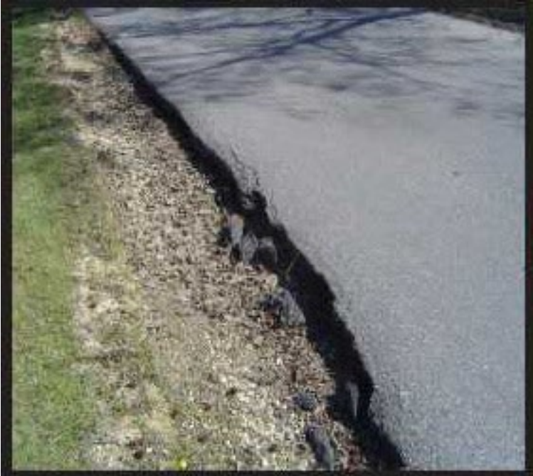
Figure A-36 High-Severity Lane/Shoulder Dropoff
