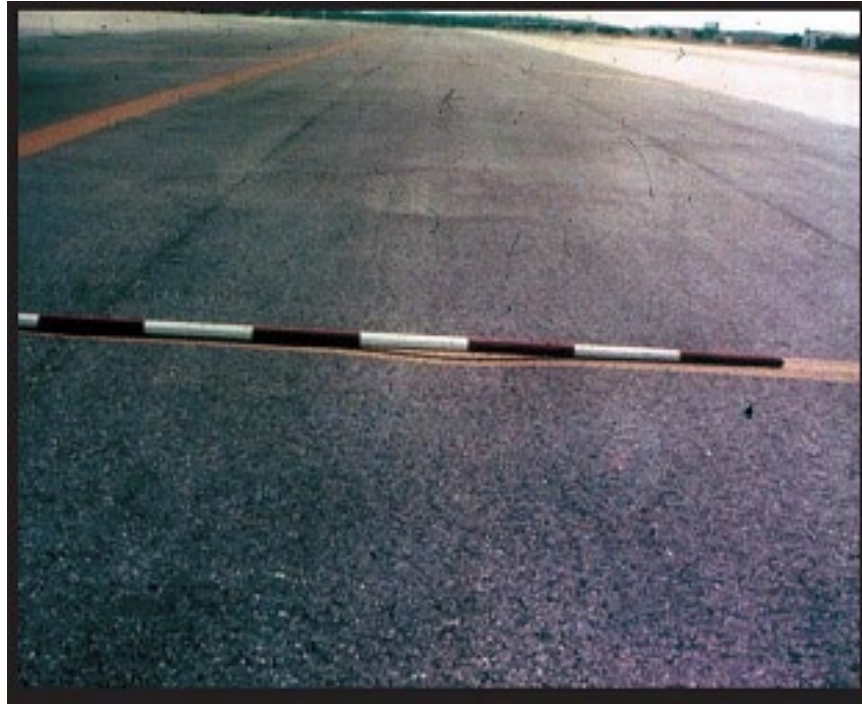
Figure A-205 Low-Severity Rutting
