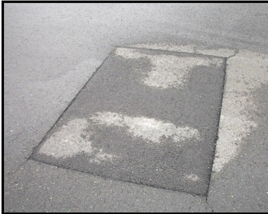
Figure A-188 Low-Severity Patching
