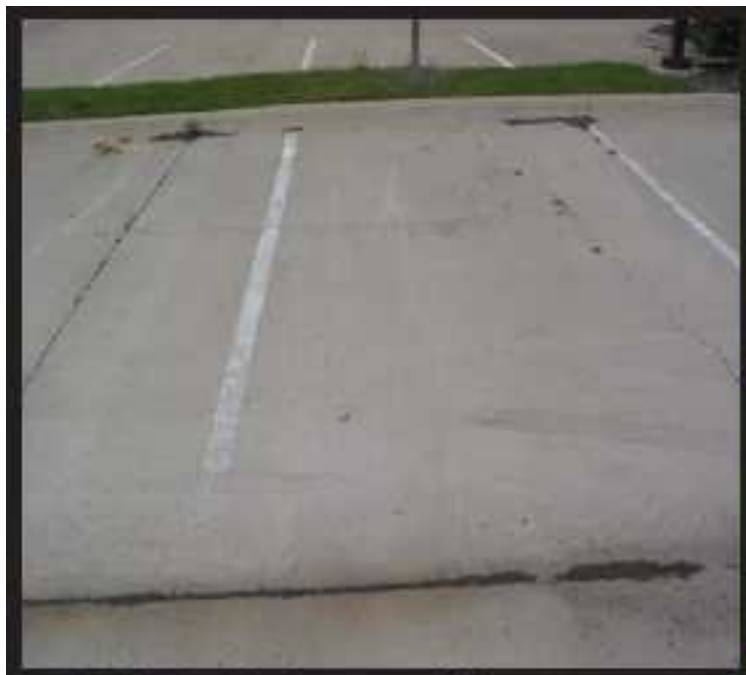
Figure A-86 Low-Severity Divided Slab
