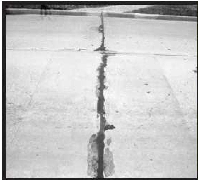
Figure A-98 Low-Severity Joint Seal Damage
