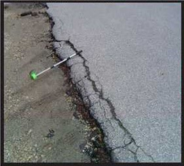
Figure A-28 High-Severity Edge Cracking
