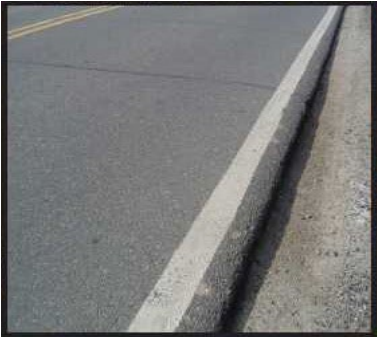
Figure A-35 Medium-Severity Lane/Shoulder Dropoff
