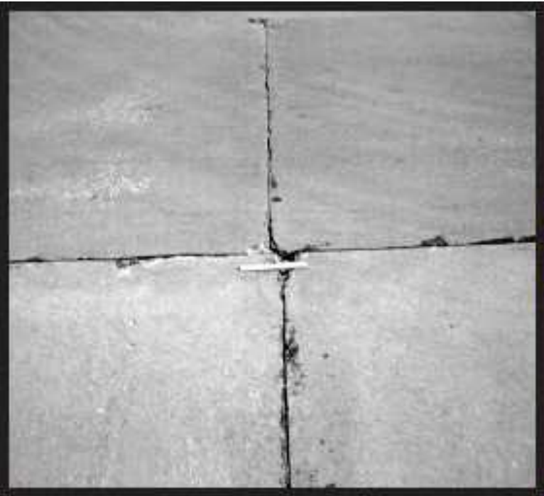
Figure A-139 Low-Severity Corner Spall
