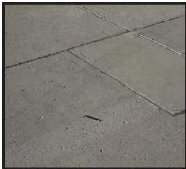
Figure A-110 Low-Severity Large Patch and Utility Cut
