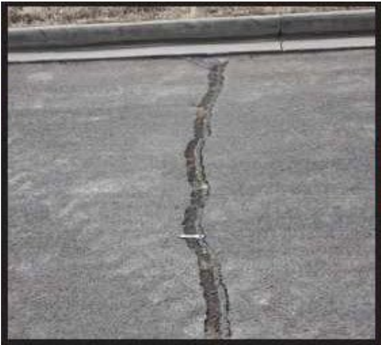
Figure A-40 High-Severity Longitudinal and Transverse Cracking
