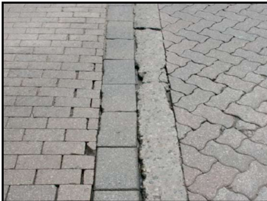
Figure A-308 Low-Severity Edge Restraint Damage
