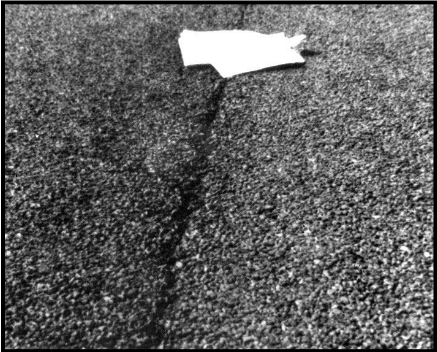
Figure A-184 High-Severity PFC L&T Cracking
