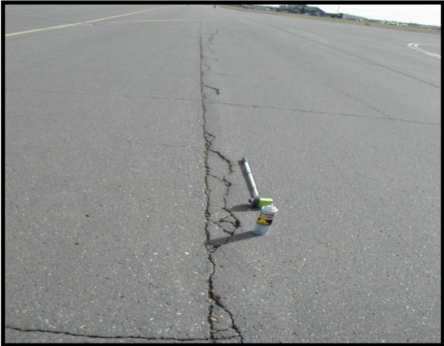
Figure A-176 High-Severity Joint Reflection Cracking
