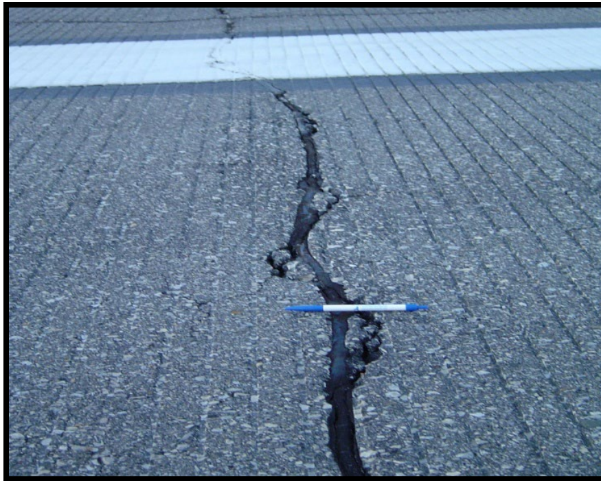
Figure A-180 High-Severity L&T Cracking
