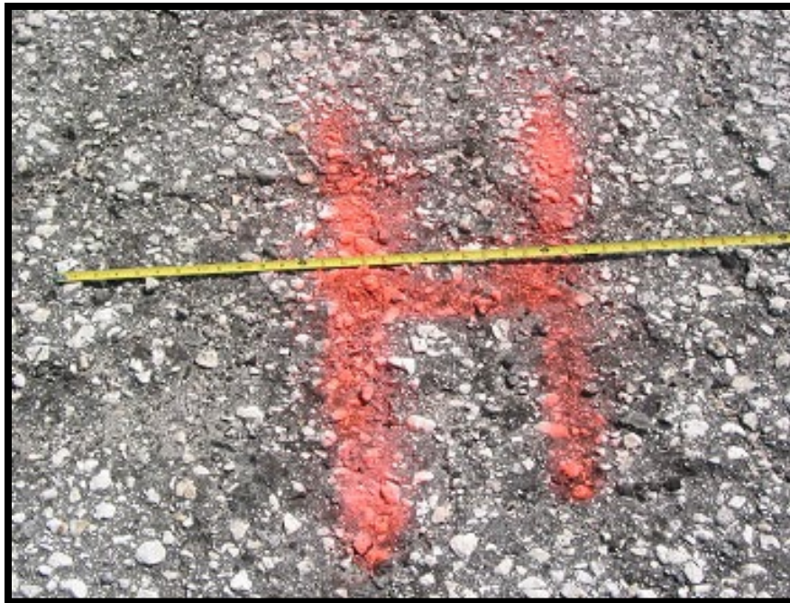
Figure A-196 High-Severity Raveling (Dense Mix)
