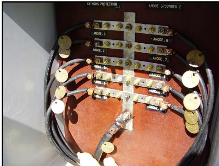
Figure B-18 Anode Junction Box
