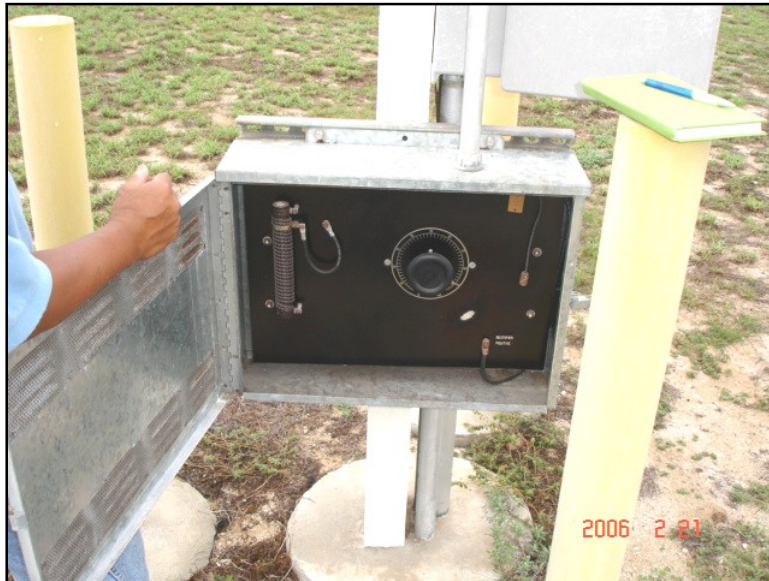
Figure B-8 Resistors in an Above Grade Terminal Box
