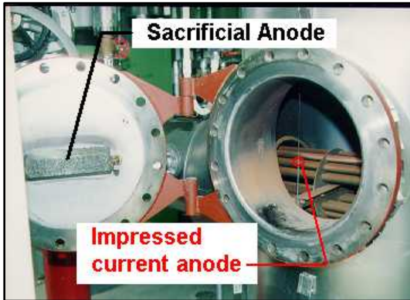
Figure B-34 CP System for a Vertical Hot Water Tank with a Man-Way Access Opening.
