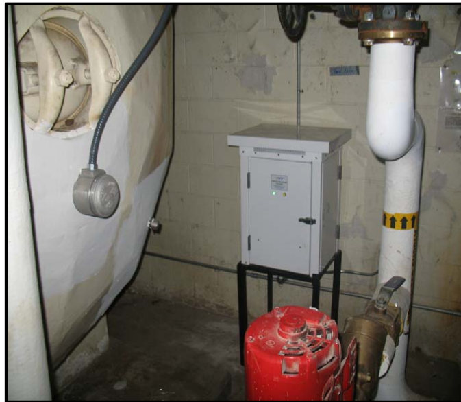
Figure B-35 CP System Rectifier and Anode Condulet Fitting on Side of Water Tank.
