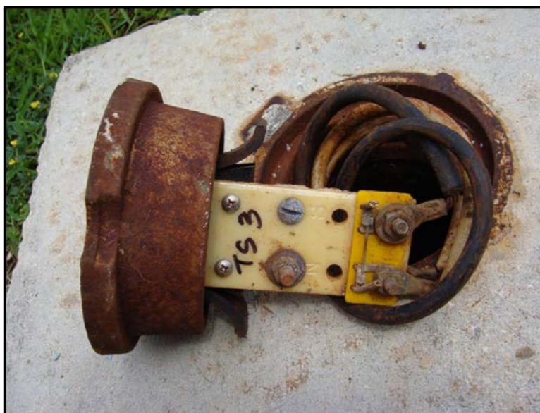
Figure B-14 Small Flush Mounted Test Station with Too Many Large Sized Wires.
