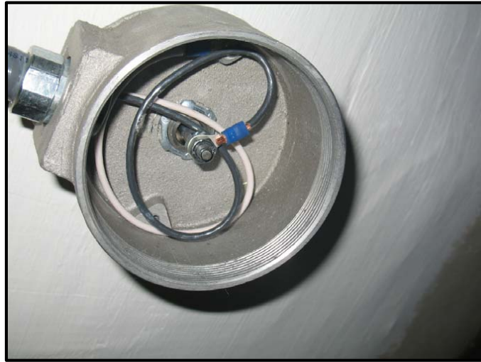
Figure B-36 Close up of Condulet Fitting Showing Anode Rod Extending Out of the Storage Tank.
