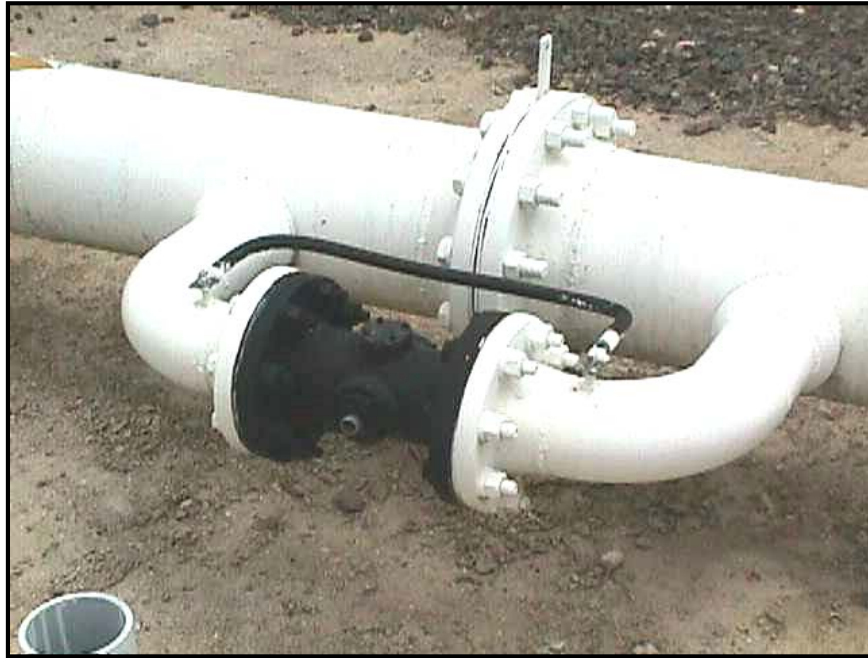
Figure 4-3 Bond Wire Installed Between Two Electrically Isolated Pipe Sections
