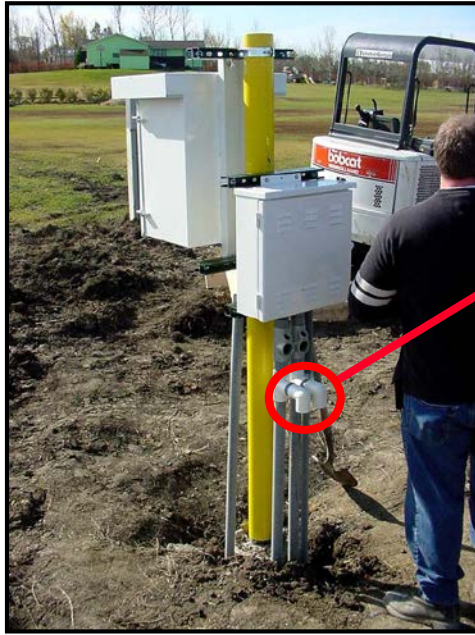
Figure B-23 Anode Column Vent Pipes Run Outside of Anode Junction Box.
