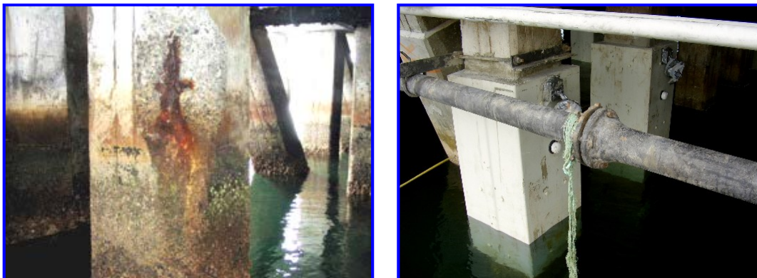
Figure B-29 Photos Showing “Before” and “After” Installation of Integrated Pile Repair and CP Systems
