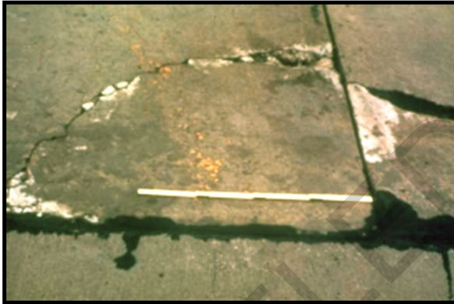
Figure B-7 High-Severity Corner Break
