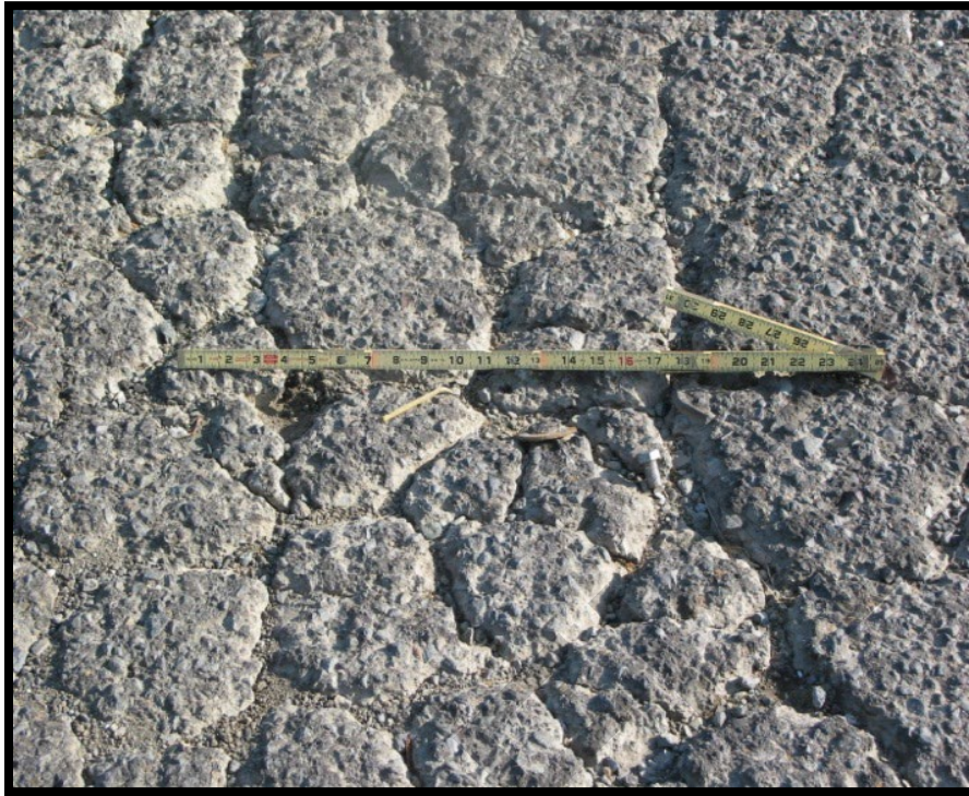
Figure A-3 High-Severity Alligator Cracking
