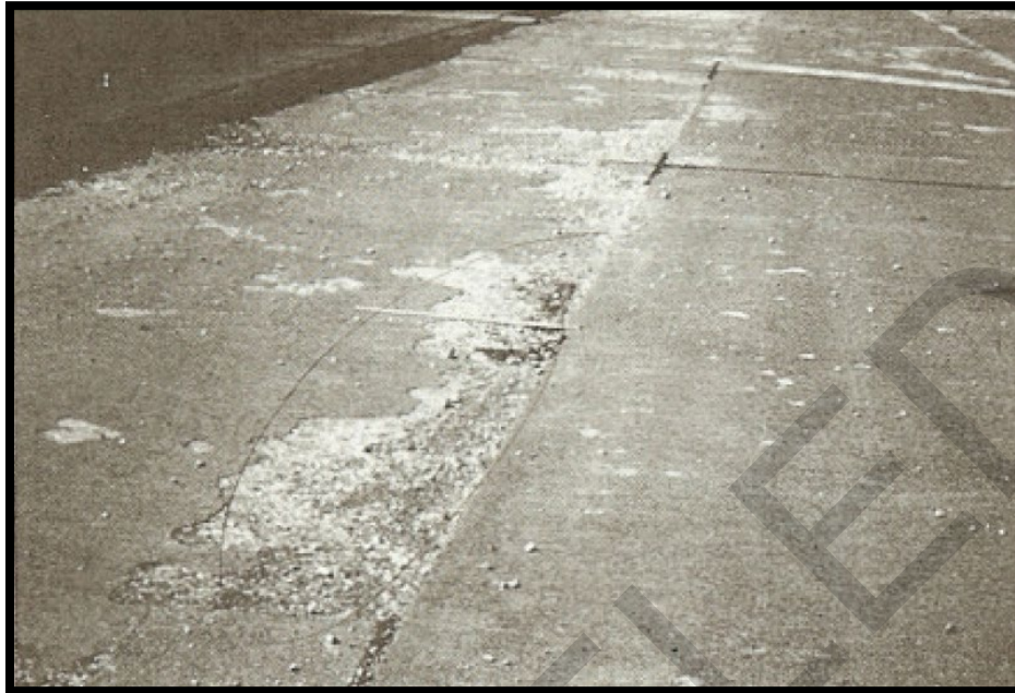
Figure B-29 High-Severity Scaling
