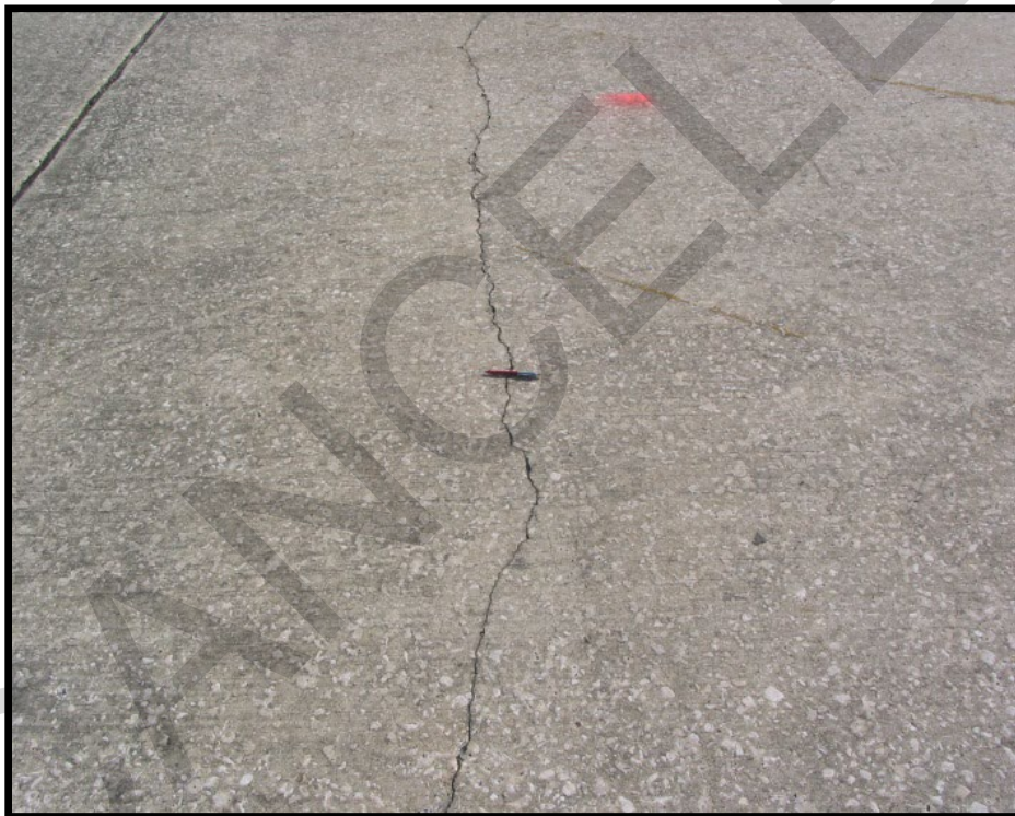
Figure B-8 Low-Severity Linear Cracks
