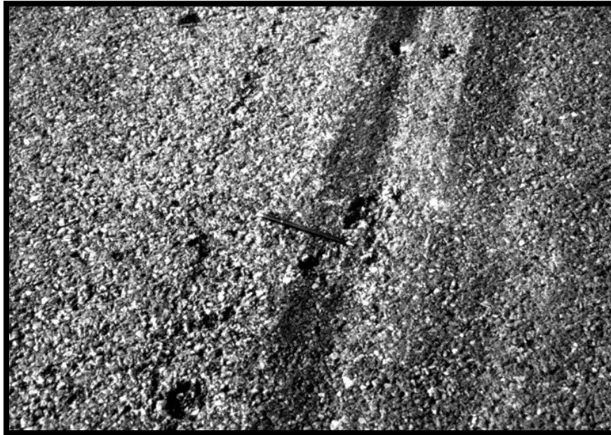
Figure A-45 High-Severity Raveling (PFC)
