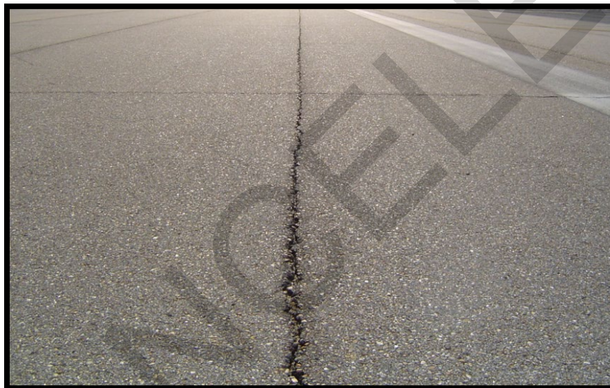
Figure A-21 Low-Severity Joint Reflection Cracking
