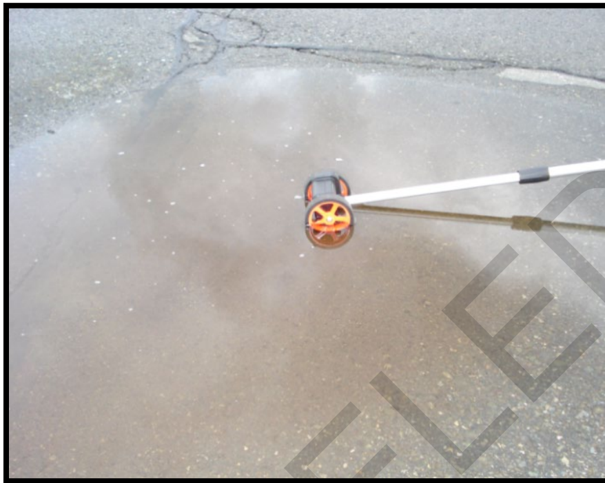
Figure A-19 High-Severity Depression
