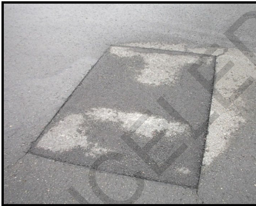
Figure A-33 Medium-Severity Patching
