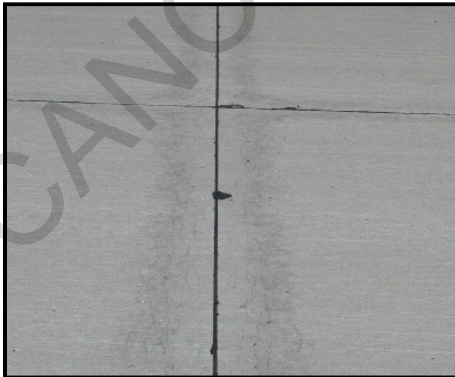
Figure B-12 Low-Severity “D” Cracking
