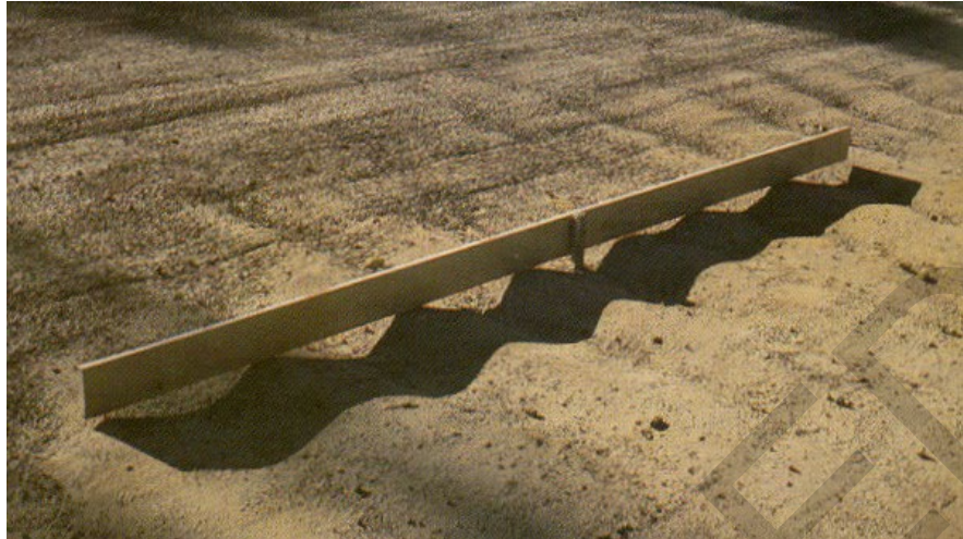
Figure A-15 High-Severity Corrugation
