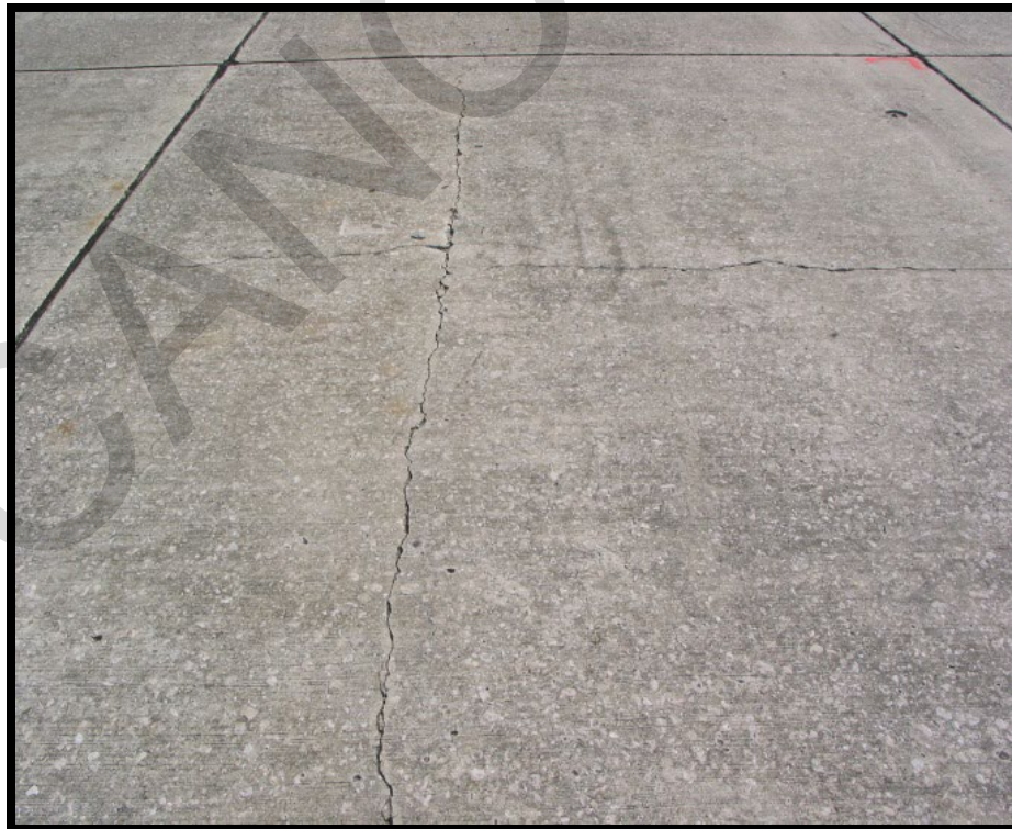
Figure B-33 Low-Severity Shattered Slab/Intersecting Cracks
