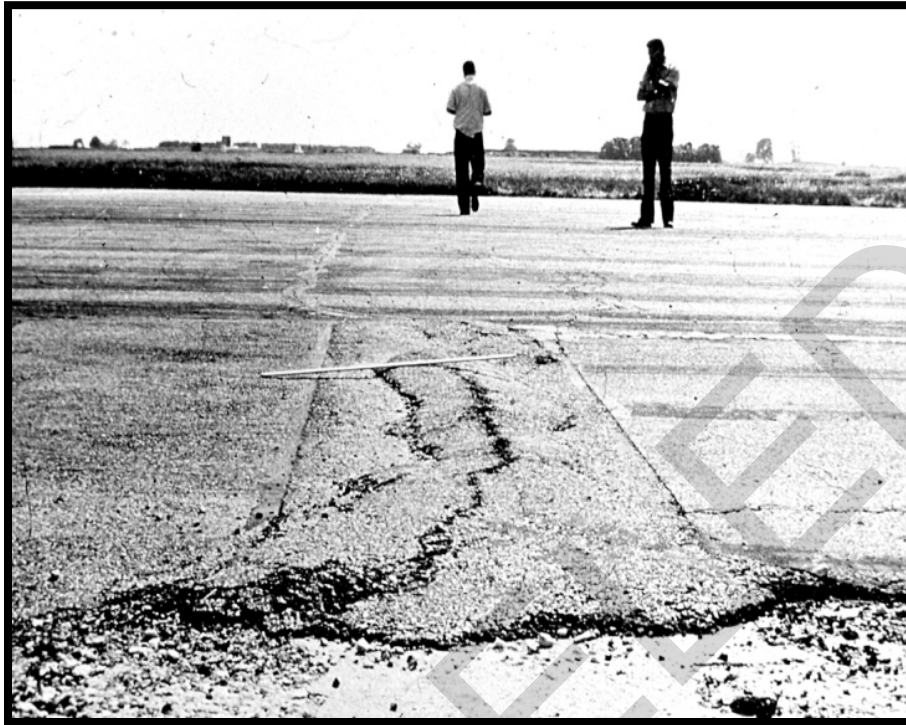
Figure A-34 High-Severity Patching
