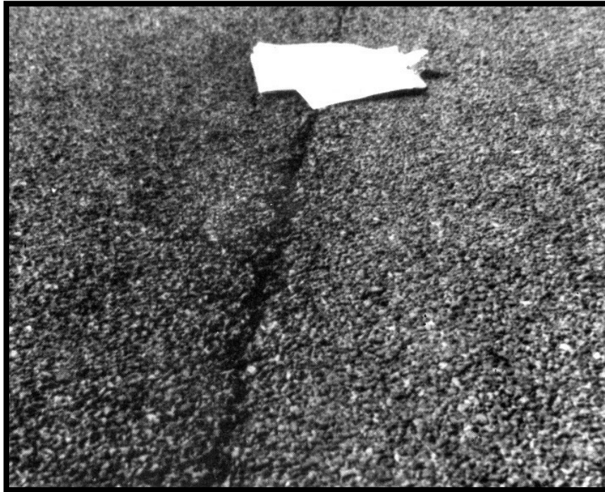
Figure A-30 High-Severity PFC L&T Cracking
