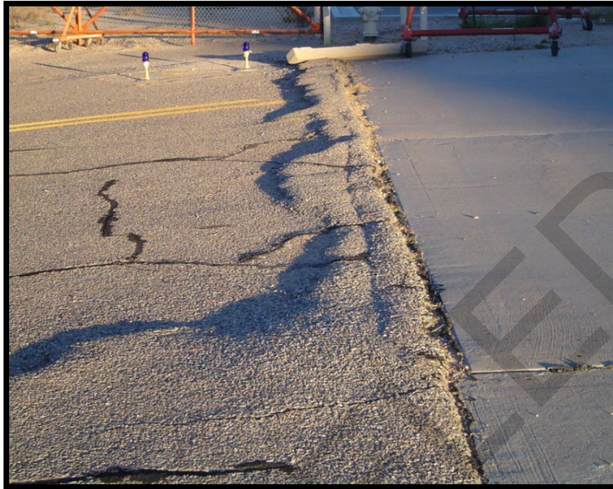
Figure A-49 High-Severity Shoving
