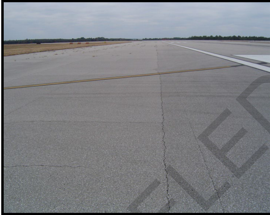
Figure A-22 Medium-Severity Joint Reflection Cracking
