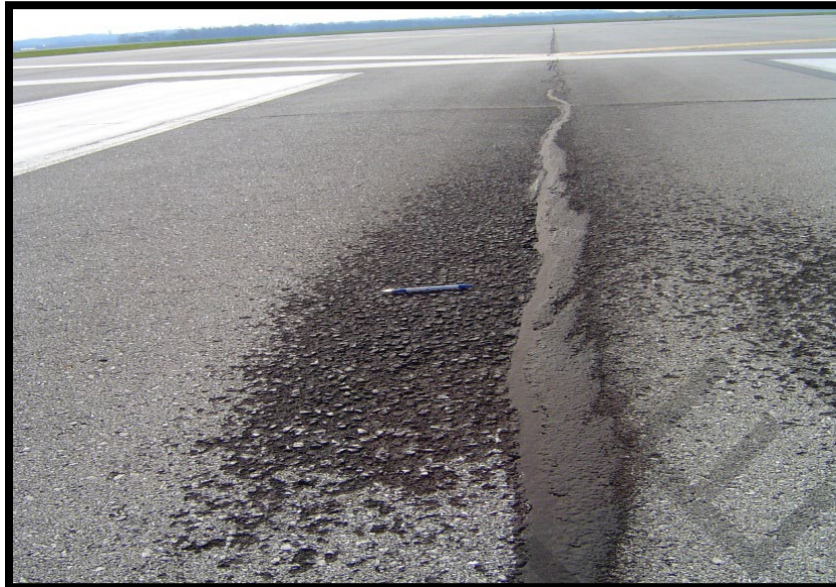
Figure A-20 Jet Blast Erosion
