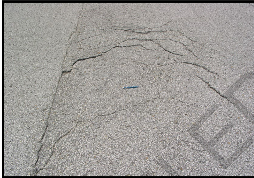
Figure A-50 Slippage Cracking
