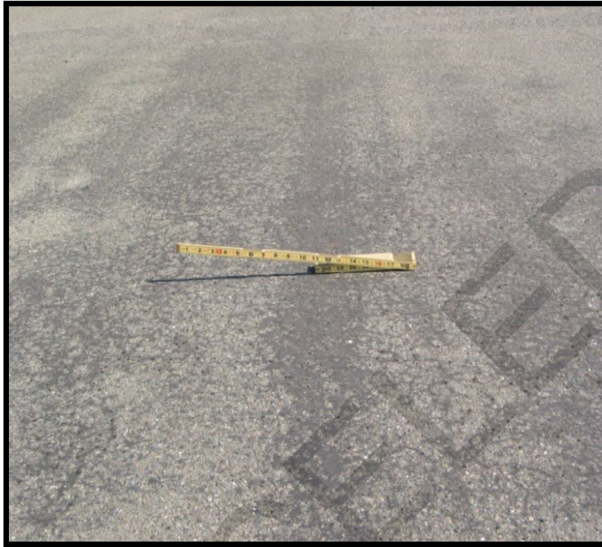
Figure A-5 Bleeding
