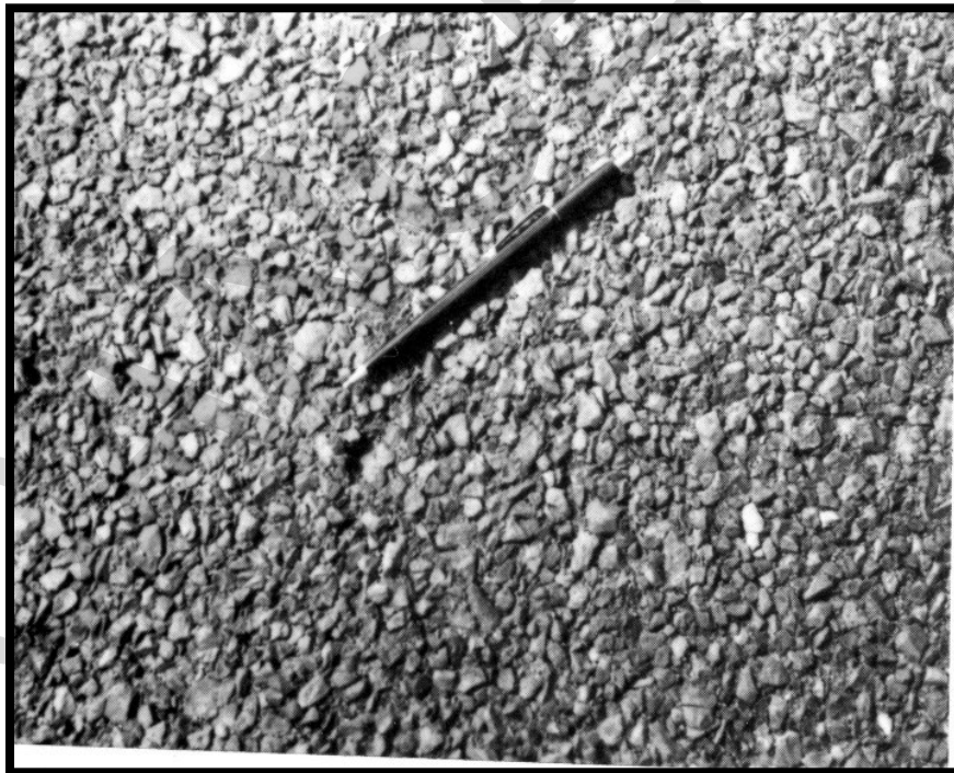
Figure A-42 Low-Severity Raveling (PFC)
