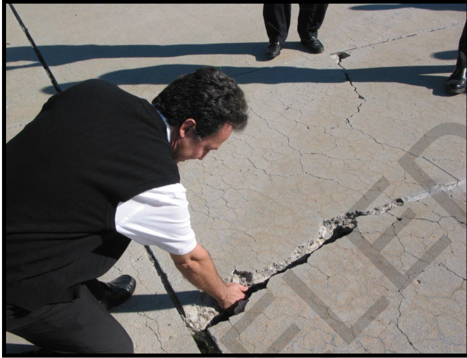
Figure B-46 High-Severity ASR
