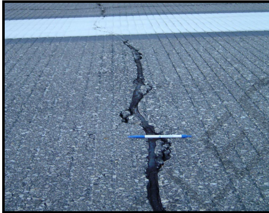
Figure A-26 High-Severity L&T Cracking
