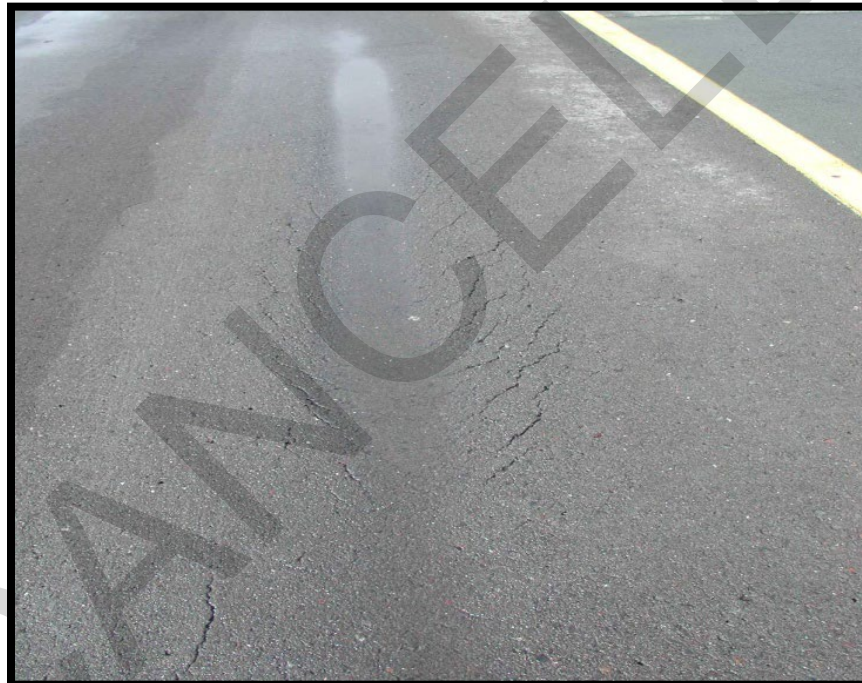
Figure A-46 Rutting
