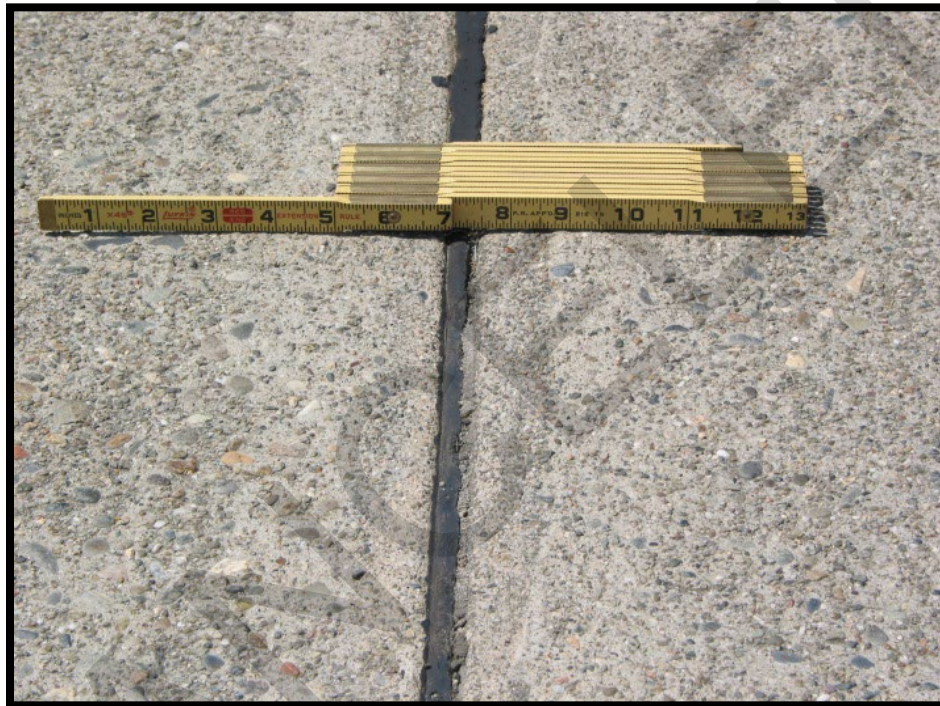
Figure B-15 Low-Severity Joint Seal Damage
