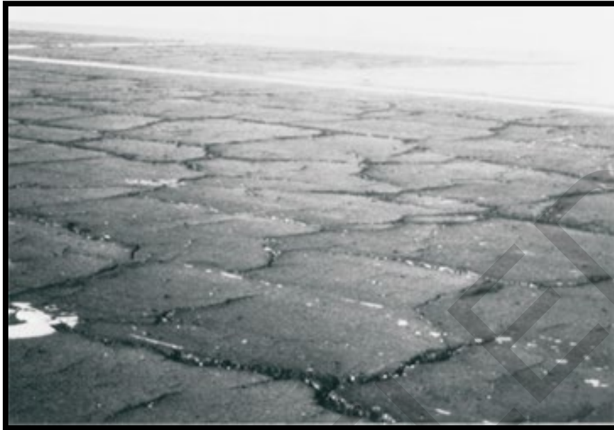
Figure A-11 High-Severity Block Cracking
