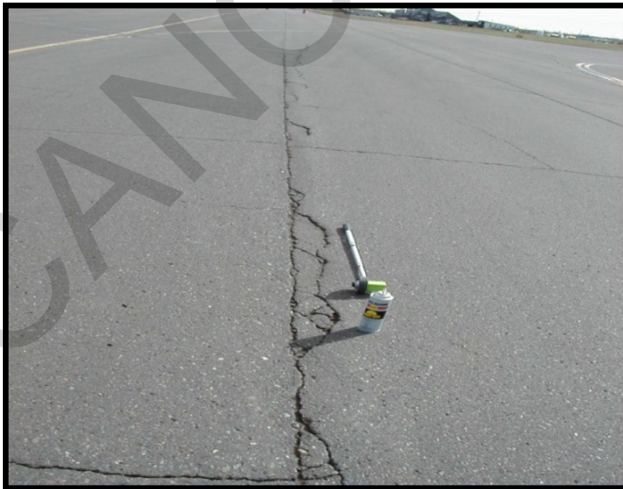
Figure A-23 High-Severity Joint Reflection Cracking
