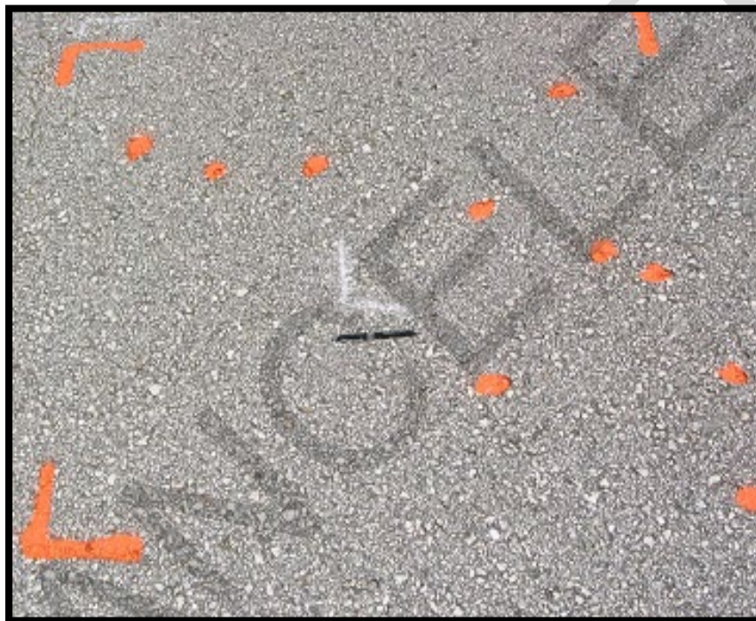
Figure A-36 Low-Severity Raveling (Dense Mix)
