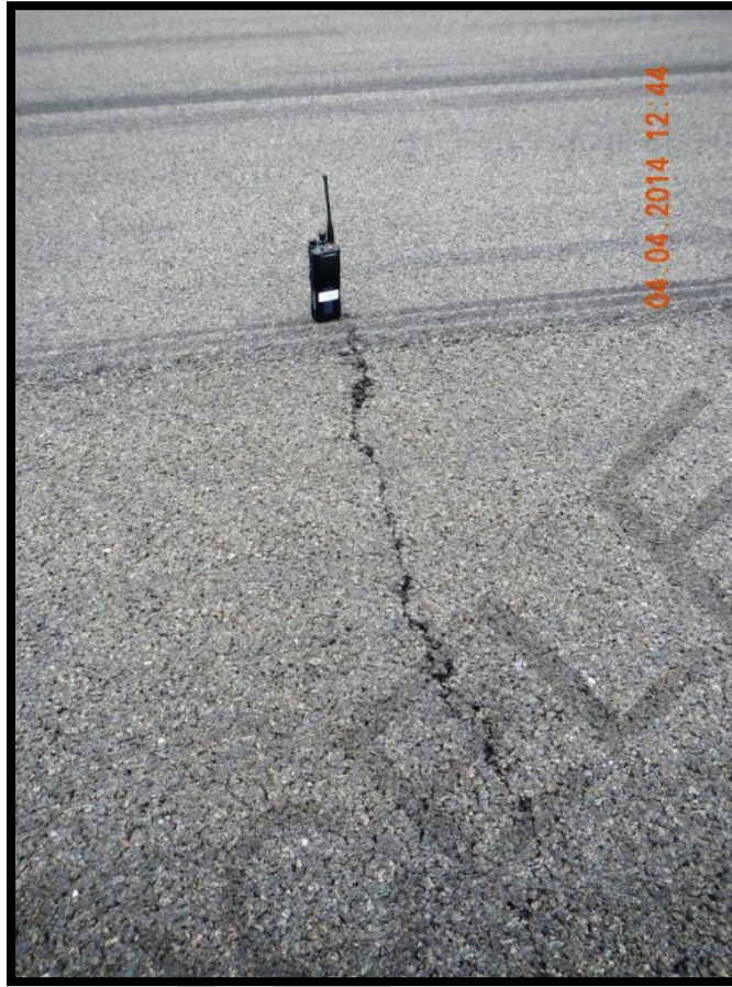
Figure A-29 Medium-Severity PFC L&T Cracking
