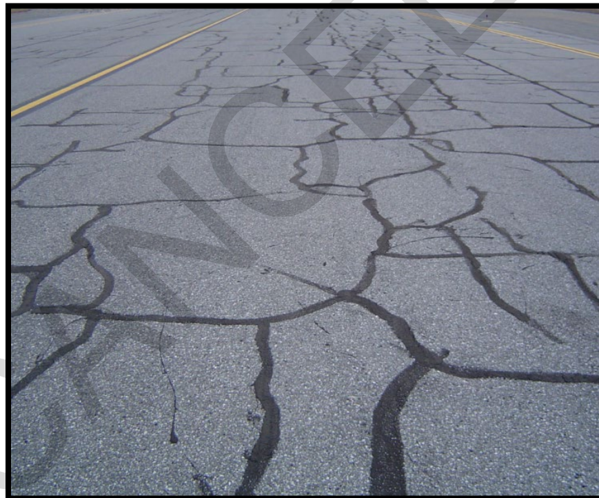
Figure A-6 Low-Severity Block Cracking
