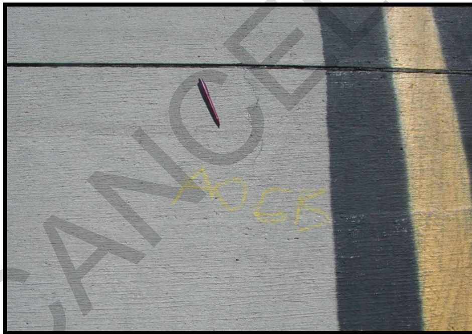
Figure B-36 Shrinkage Cracks
