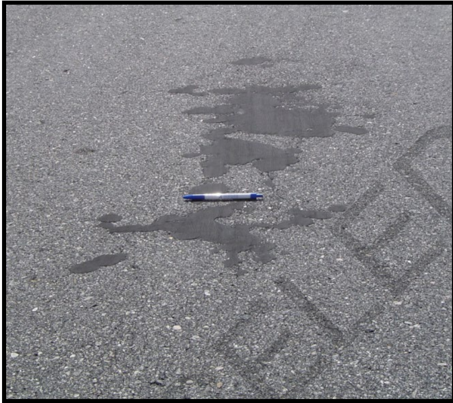
Figure A-4 Bleeding
