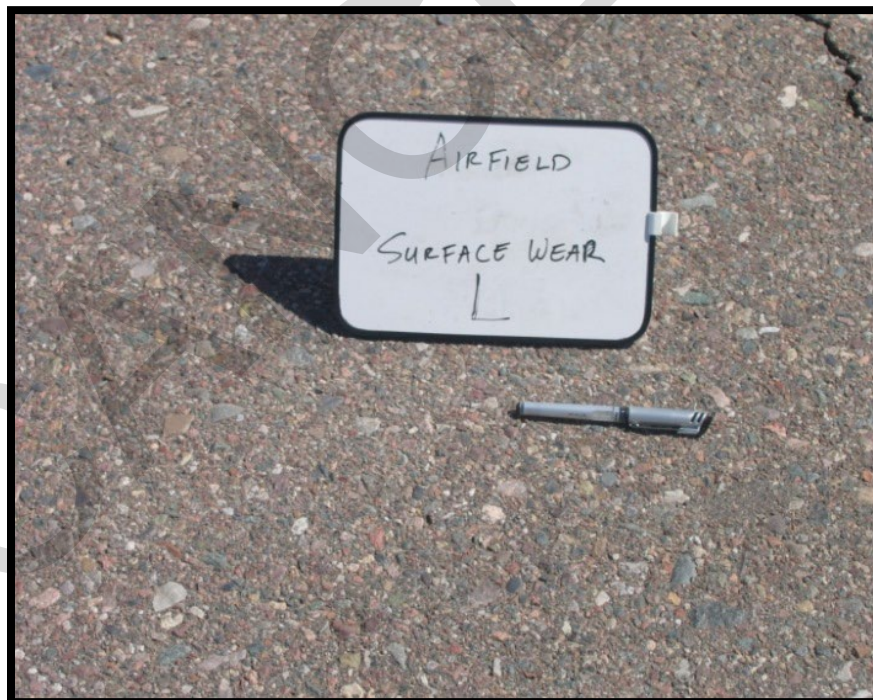
Figure A-54 Low-Severity Weathering
