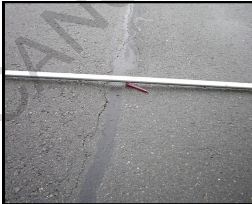
Figure A-16 Low-Severity Depression
