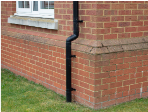
Downspout to Underground Drainage
