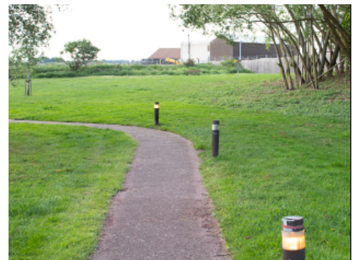
Bollard Lighting at Trail
